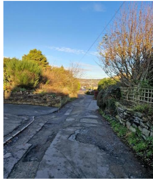
Photo 8: Privately maintained section of Colders Lane for private carriage access to residential properties. Uneven surface with several layers of tarmac.
