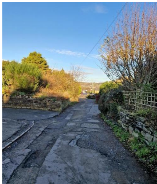
Photo 8: Privately maintained section of Colders Lane for private carriage access to residential properties. Uneven surface with several layers of tarmac.
